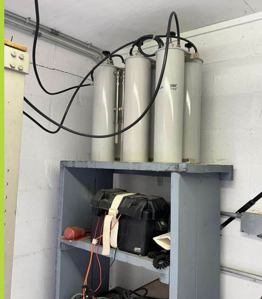
VHF Duplexer & Battery Backup
