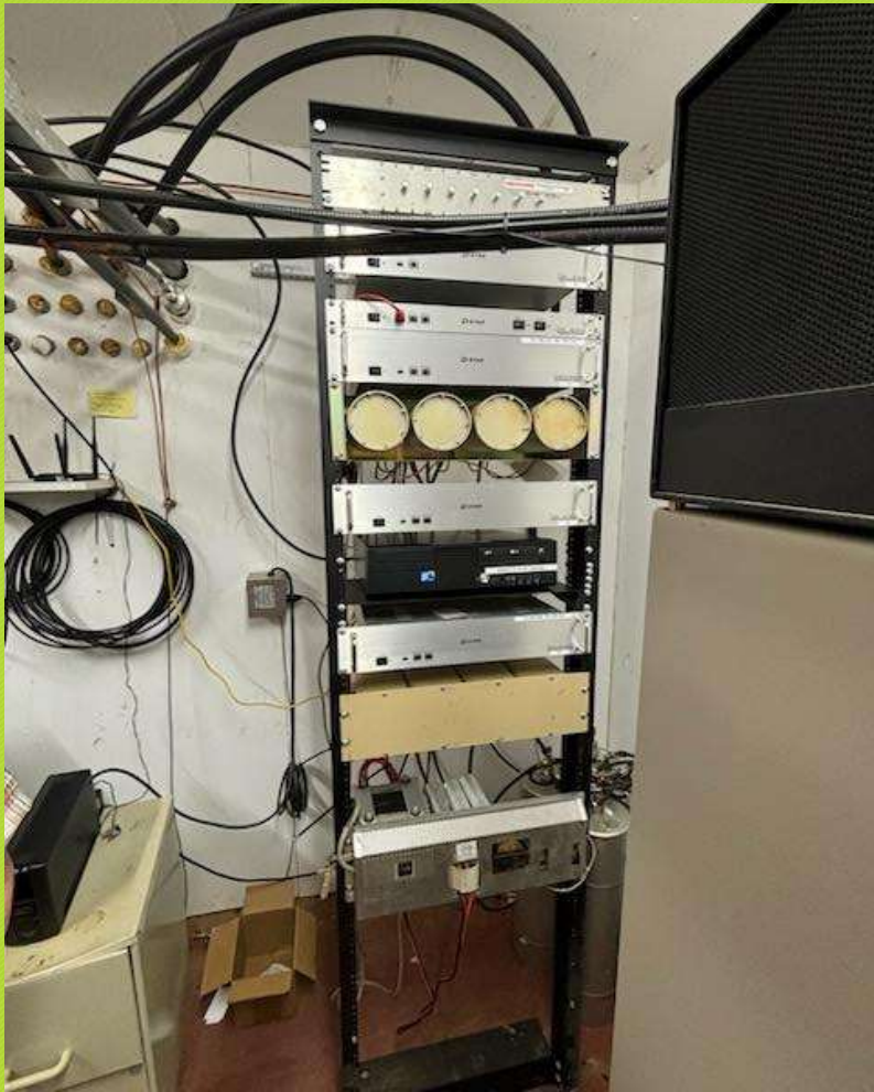
DSTAR Repeater Rack
