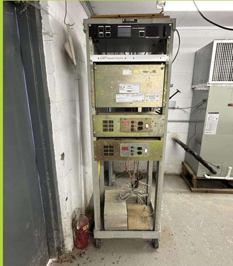
N4MZ VHF Repeater Rack
